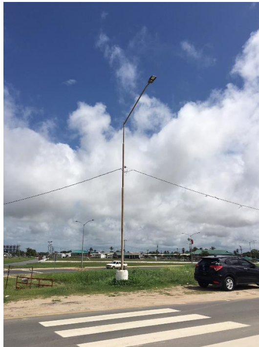
Installed LED Lamp
