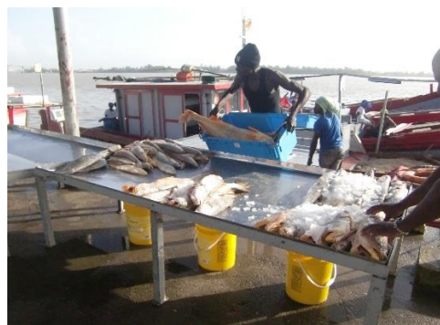
Unloaded fish being preserved by ice produced by the ice-making machine installed by Japan's grant aid.
