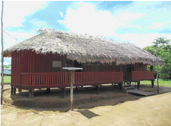
Photo of the renovated health clinic in Pelelu, Tepu, funded by the Government of Japan's GGP scheme.
