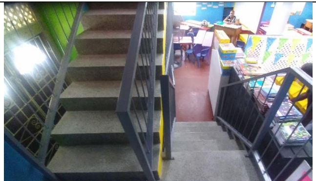
New staircase and banister, which were included as part of the renovation
