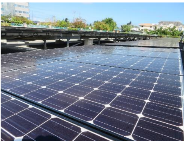
Installed solar panels
