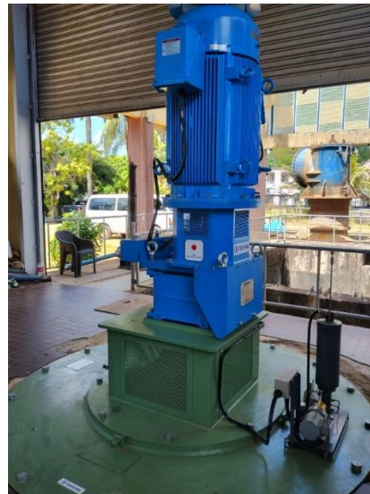
Display of the newly installed drainage pumps.
