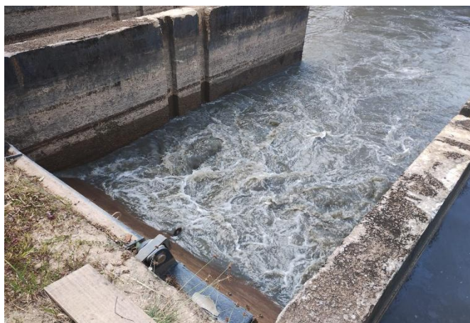
Water being discharged from the drainage pump station.
